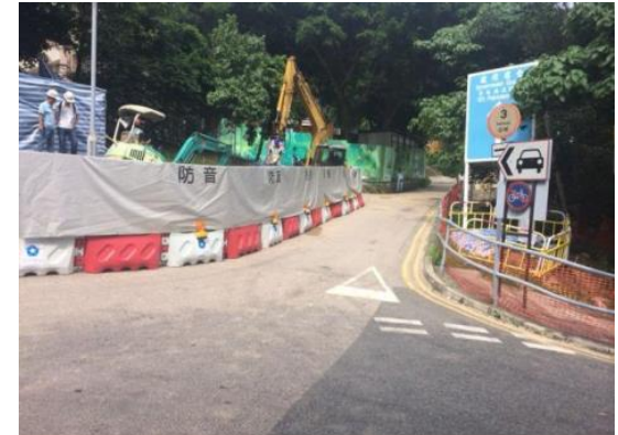
Extensive noise barriers
