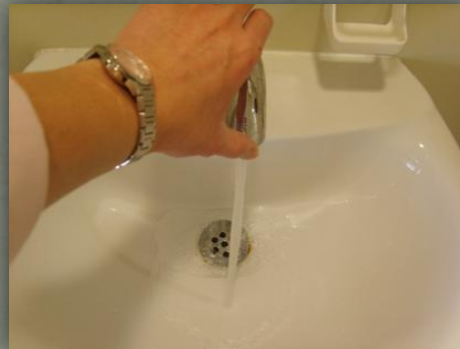
Add water to floor drain and sink
